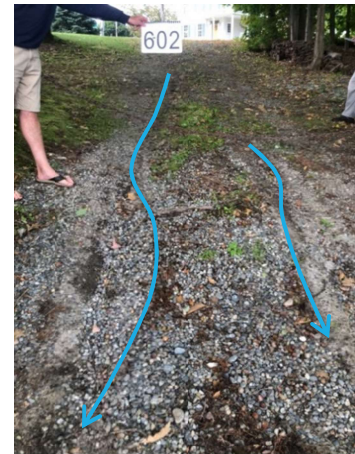
Medium impact erosion site 6-02 on a residential boat access.
