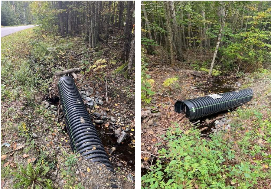
High impact erosion site 3-04 on N. Wayne Road in North Wayne. Snowmobile trail cross-culvert failure.
