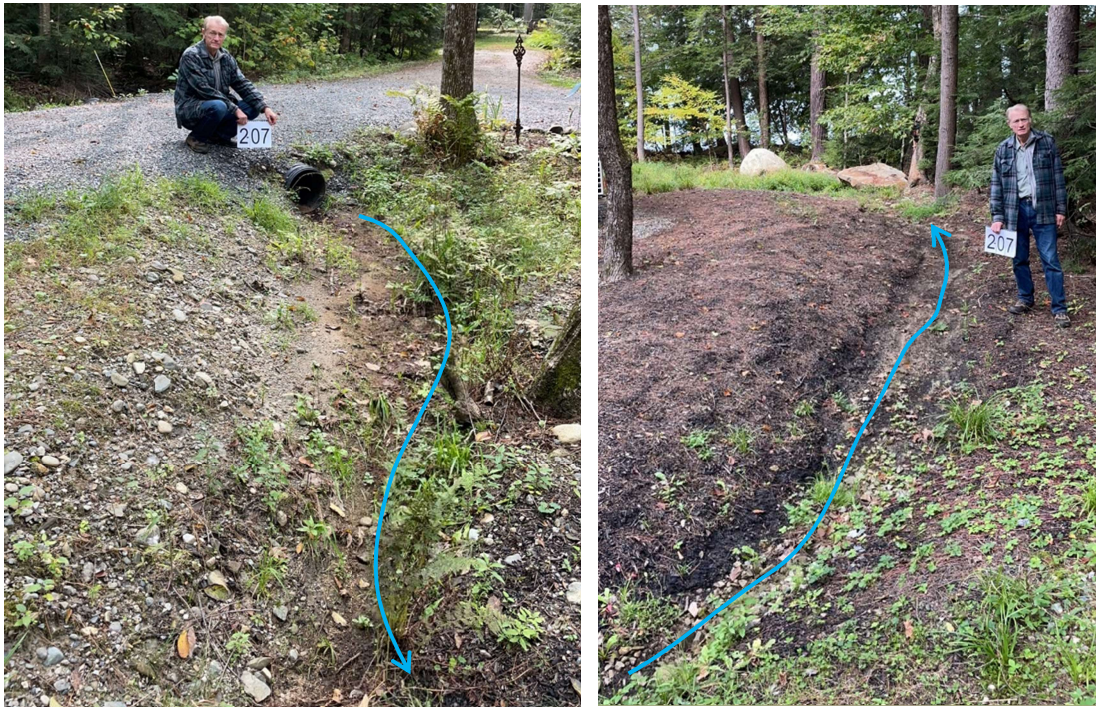
High impact erosion site 2-09 at a residential property with surface erosion (rill) and bare soil on a driveway leading down to water access.
