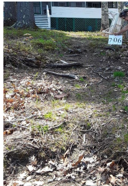
Surface erosion on a pathway leading to Androscoggin Lake.
