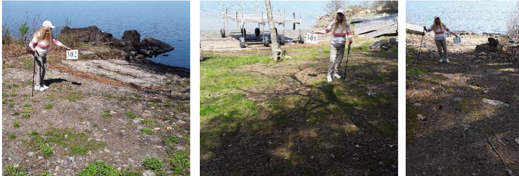
Examples of sites identified in Sector 3: Site 3-02 (left) erosion on a beach access, site 3-08 (middle) bare soils and sheet erosion over a lawn without a shoreline buffer, and site 3-13 (right) erosion documented on a shorefront path.
