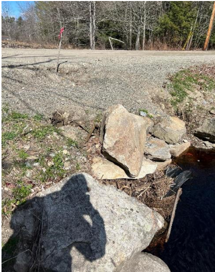
Site 4-01 in Wilson Pond Road in Monmouth – crushed culvert inlet.
