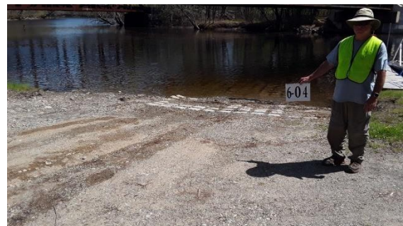
Erosion documented at a commercial boat launch in Sector 6 (site 6-04).
